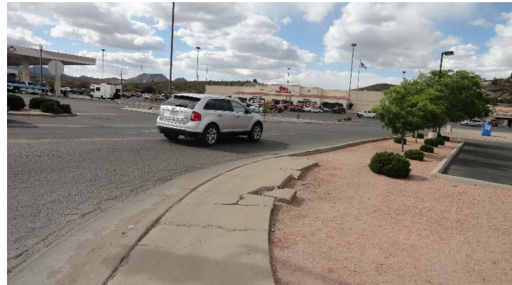
Figure 5: Sidewalk deterioration and ending looking towards Globe Food Mart.
