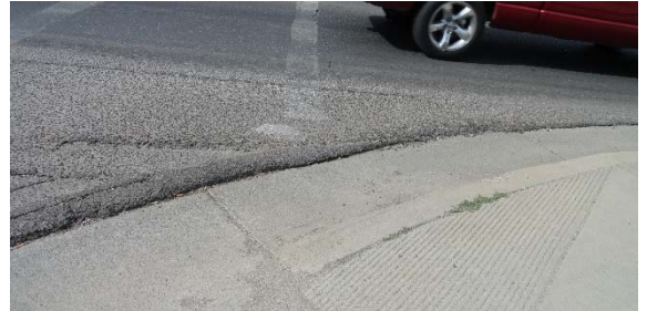
Figure 4: Asphalt Next to Gutter Lip being pushed and causing a trip hazard.
