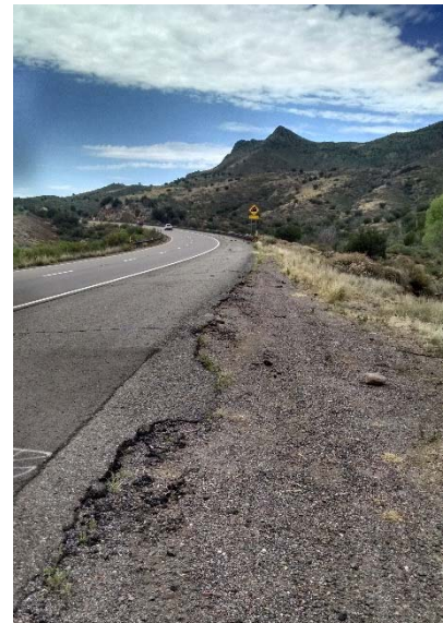
Figure 33: Eroding edge of roadway
