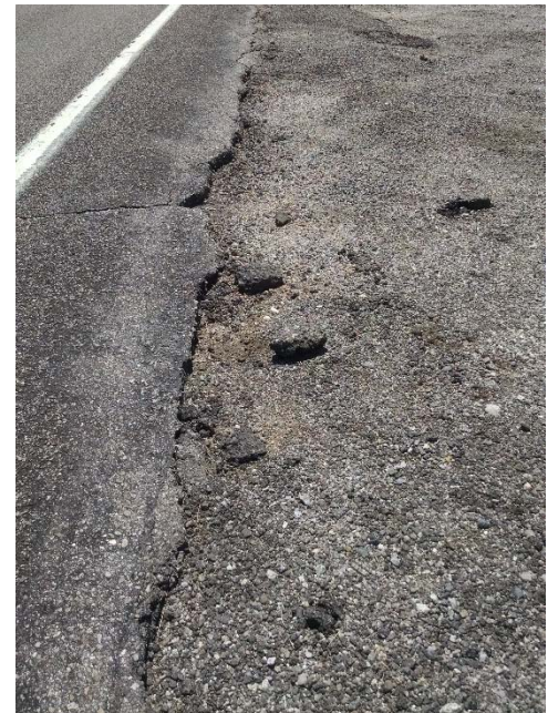
Figure 43: Edge of roadway eroding.
