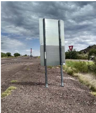
Figure 34: Sign near intersection of SR 87& SR 188. Improper mounting height and breakaway base.
