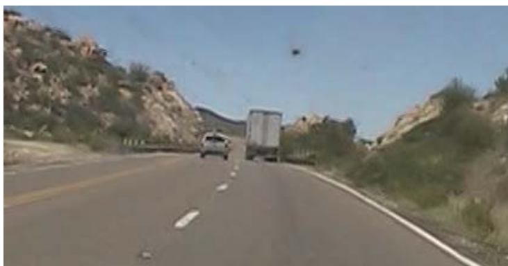
Figure 45: Faded Striping & Small Shoulder
