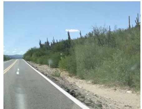
Figure 38: Eroding edge of travelway.
