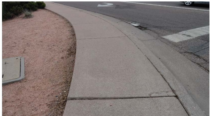
Figure 11: Sidewalk edge drop-off
